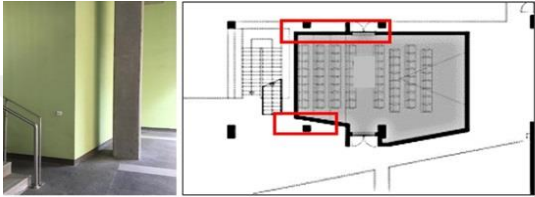
Figure 92. The gap between the column and the wall (Photo by: Seyedalipour, 2020)
