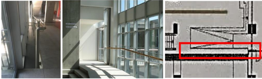
Figure 64. The gap between the ramp and the façade (Photo by: Seyedalipour, 2020)
