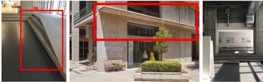
Figure 86. Left (A): angular relationship between the ramp and the stairs; middle (B): protrusion of the concrete slabs; right (C): white part of the ceiling (Photos by: Seyedalipour, 2020)
