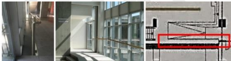
Figure 50. The gap between the ramp and the façade (Photo by: Seyedalipour, 2020)
