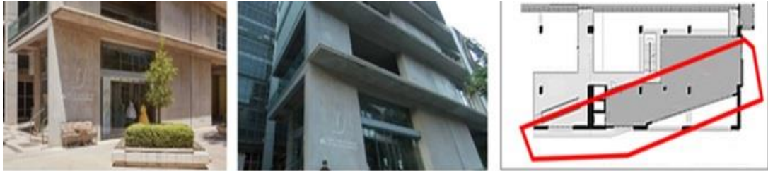
Figure 62. The protrusion of the concrete slabs as a habitable poché (Photo by: Seyedalipour, 2020)
