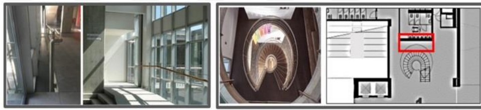
Figure 90. Left to right: (A): the gap between the ramp and the façade; (B): the gap between the restroom wall and the staircase (Photo by: Seyedalipour, 2020)
