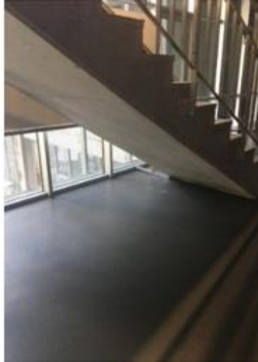
Figure 54. The triangular shape between the floor and the staircase (Photo by: Seyedalipour, 2020)
