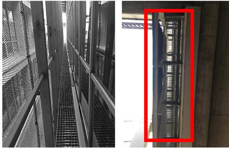
Figure 72. The gap between the double-skin façade as the second type of negative space (Photos by: Seyedalipour, 2020)
