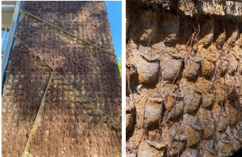
Figure 22. The D-block of Izmir University of Economics in Izmir is an example for façade integrated green wall that failed due to poor maintenance. Left, general view; right, detail of the soil pockets. (Photo taken by author on September 2022)
