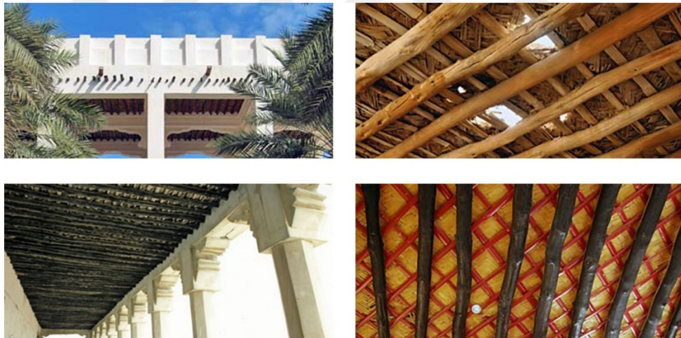
Figure 109. the traditional Arab housing the ceiling decorative elements, the images show an example from Qatar. (Source: Lockerbie, 2021)
