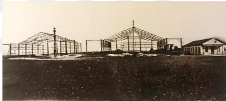
Figure 2: Construction of CIDNA facilities in 1926 (Source: Sarıgöl, cited in Hürtürk and Kline, 2009)
