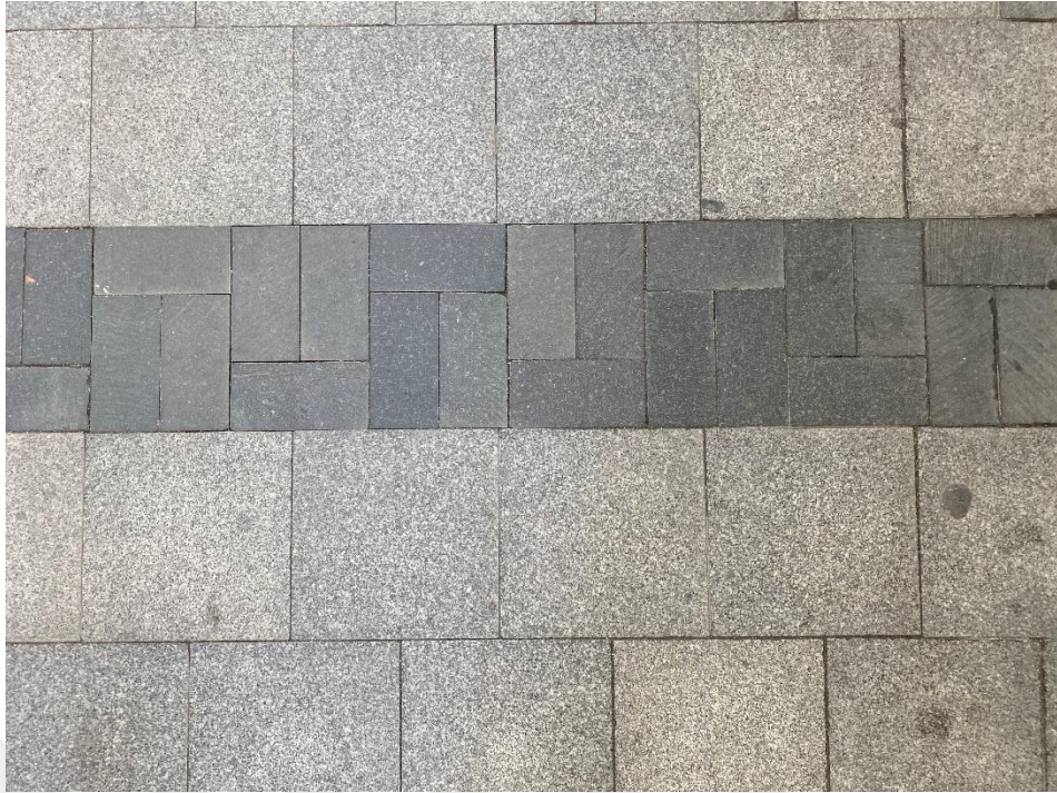
Figure 17. Flat pavement in 1476th Street
