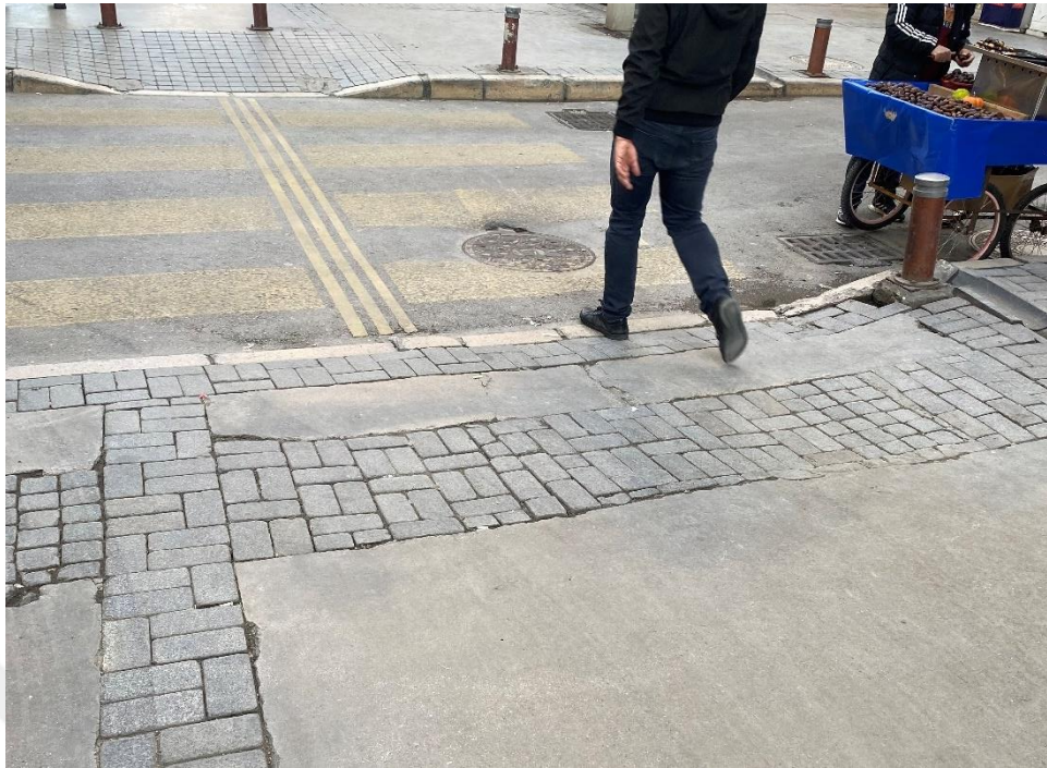
Figure 62. Slope in Kıbrıs Şehitleri Street
