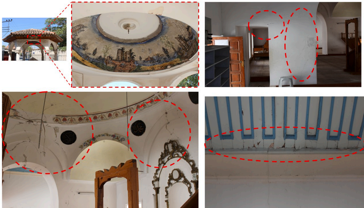
Fig. 6. Case study 1: Serious crack inside the structure and other deformations.
