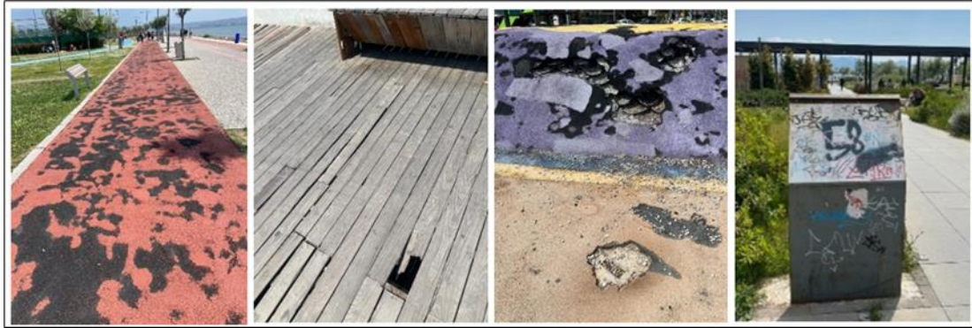
Figure 40. Some images of worn and deformed areas along the coastline (Source: photographed by author)
