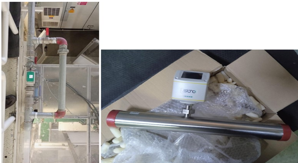
Figure 22. Flowmeters (Source: Case Study Data From the Company)
