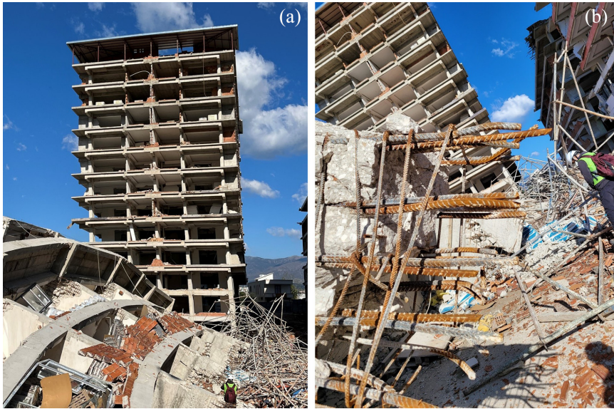
Figure 15. Building complex in Antakya: (a) building complex still standing with an approximate residual drift of 6% in the first story, and (b) identical structure that had collapsed (seen in the foreground of Figure 15a)
