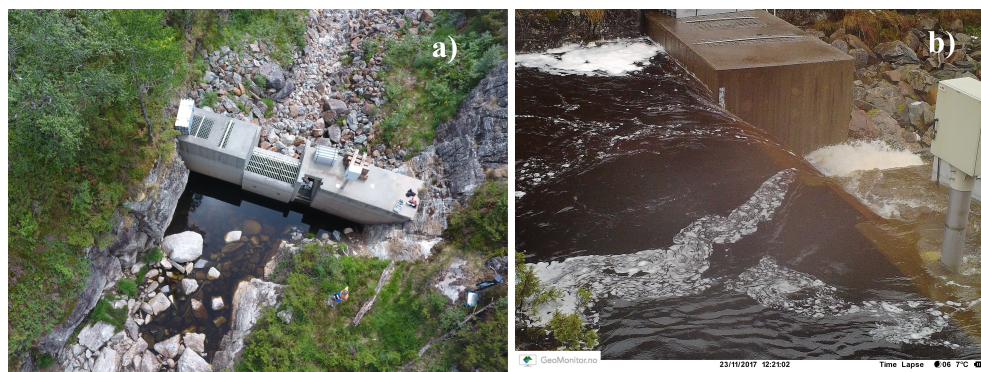
Figure 1. Downstream view of Stigansåni brook intake during (a) dry conditions and (b) wet conditions.
