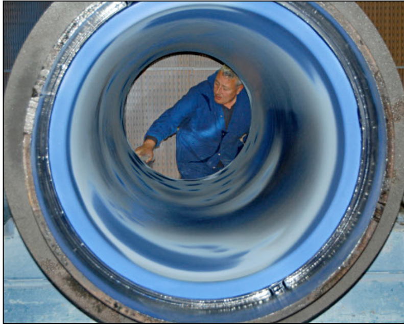
Fig.4.36: Enameled industrial lining at Pfaudler Balfour Plant. (Source: http://www.iom3.org/content/vitreous-enamel-industrial )
