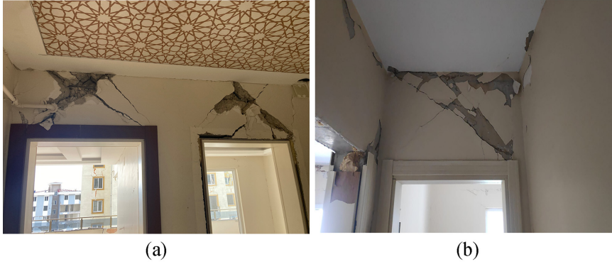
Figure 10. Shear failures in coupling beams of RC wall structures: (a) From the building in Kahramanmaraş given in Figure 8. (b) From the building in Hatay given in Figure 9d.
