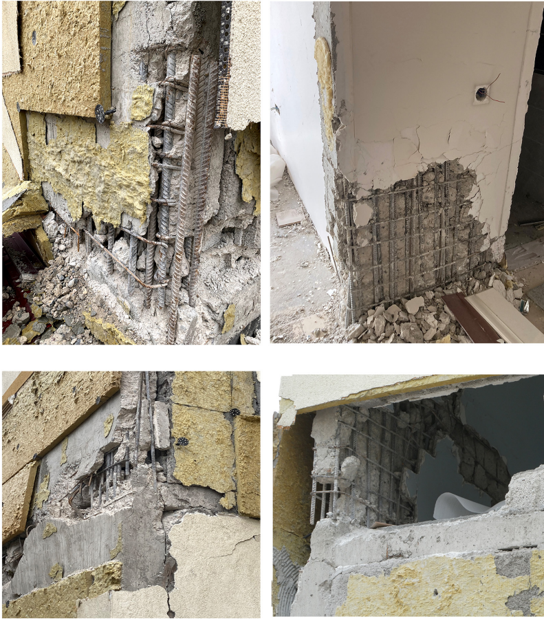
Figure 11. Lap splice damage in RC shear walls.
