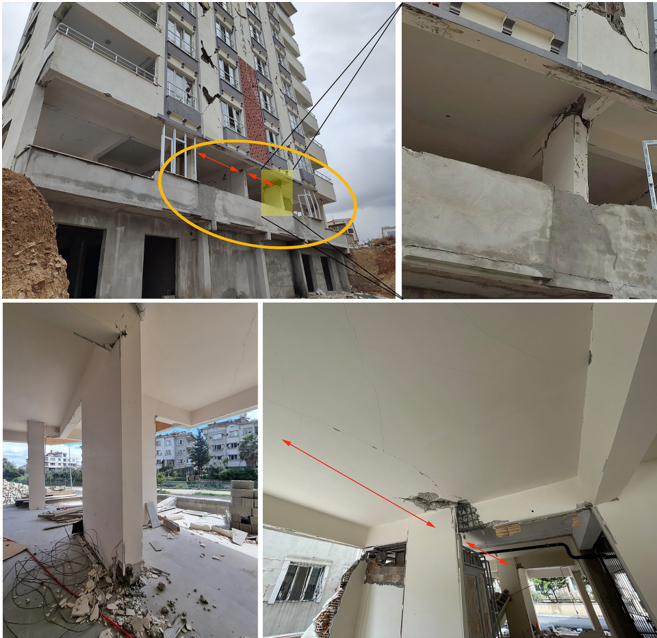
Figure 7. Damaged structural elements due to frame discontinuity.
