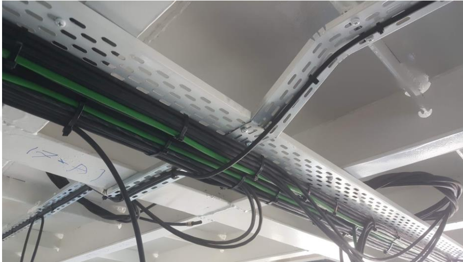
Figure 44. Electric Cable Way inside of a Steel Motor Yacht
