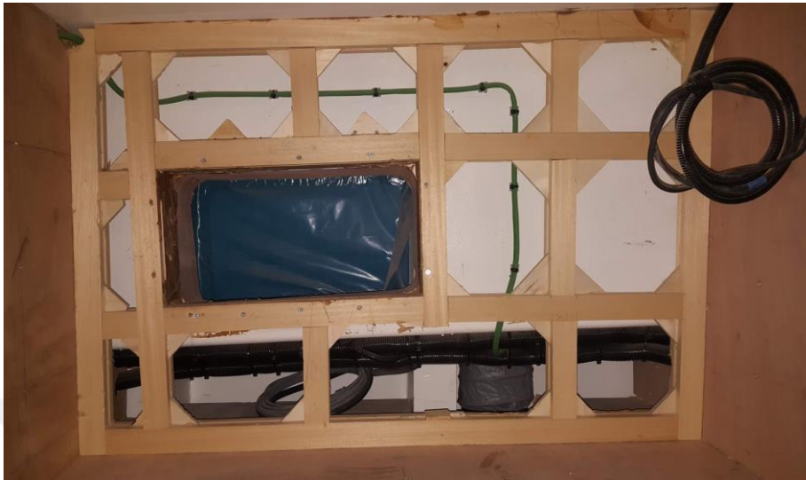
Figure 33. A Lower Deck Porthole that is Covered with Unfinished Wooden Framework
